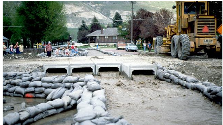
Figure 4 Sandbagging in Provo during the 1983 floods
