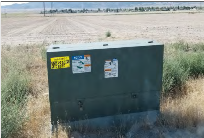
Picture 11 – Pad mounted transformers were observed along North Lake Mountain Road.
