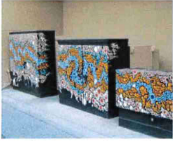
Artfully decorated utility transformers.
